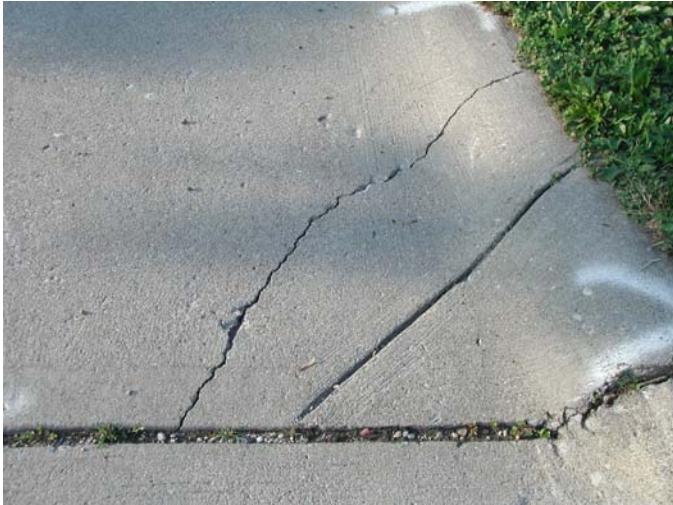
Figure 2: Zoom View of Crack and adjacent Design Groove.
