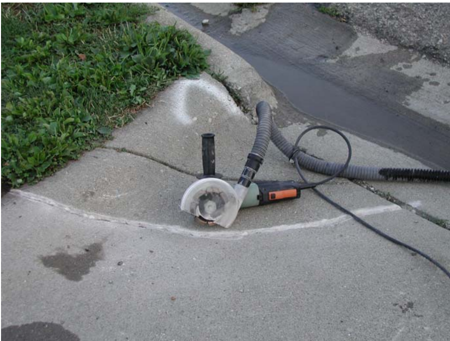
Figure 5: V Shaped Groove with Crack Sealer Segment Blade shown.
